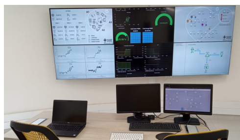
Figure 7. UPB microgrid control room.
